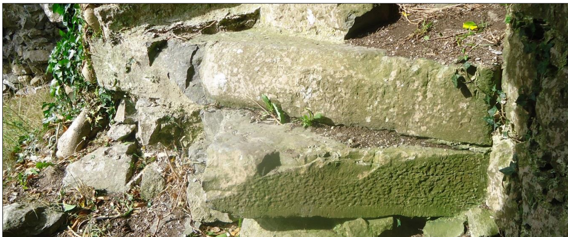
Plate 47: Ballintober Castle, northwest corner tower, detailed view of base of steps showing punch-dressing on lower step
