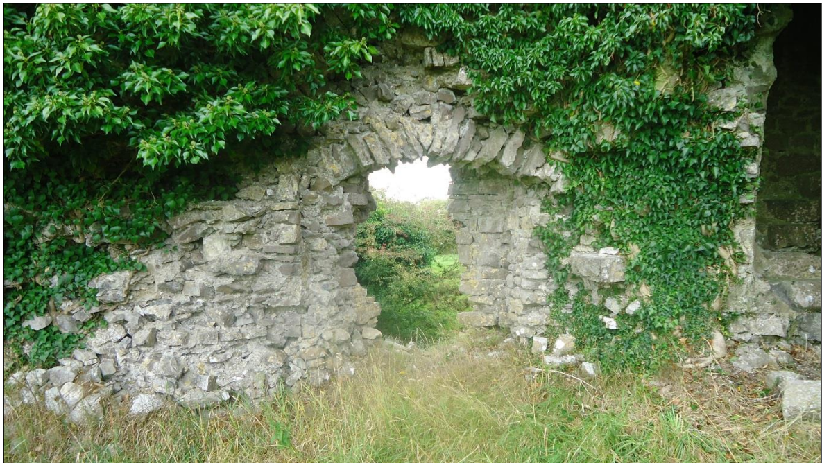
Plate 13: Ballintober Castle, view looking at interior of west wall on the north side showing remnant of window opening under arch
