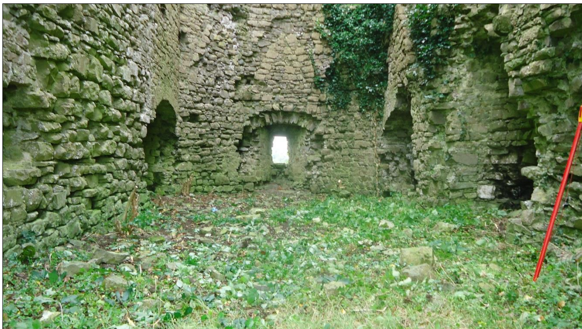
Plate 22: Ballintober Castle, southwest corner tower, view looking at ground floor window in south wall. Note too the arch-shaped feature above the window, which is related to the ceiling structure of this level
