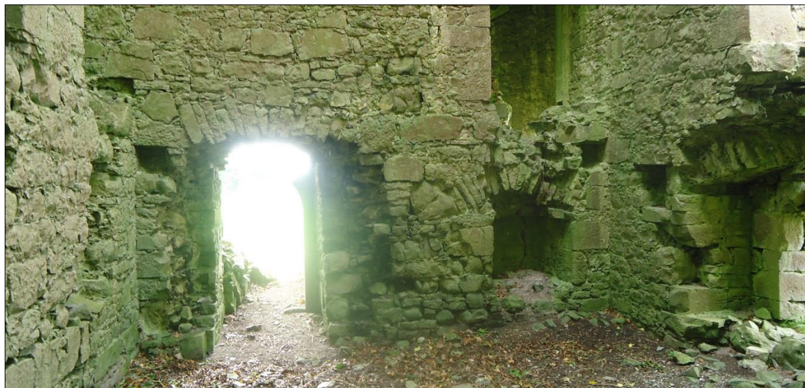
Plate 45: Ballintober Castle, northwest corner tower, view showing the ground floor looking south towards the entrance. The joist-recesses for the first-floor above are evident on the south wall of the main chamber
