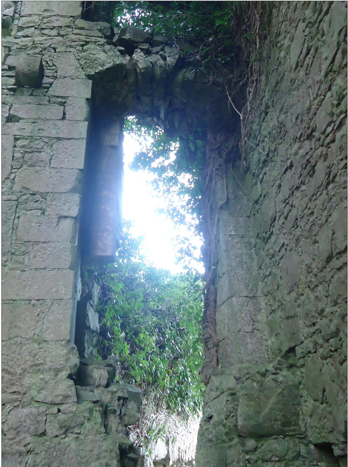
Plate 50: Ballintober Castle, northwest corner tower, view of the east-facing window opening in the first floor, suggesting the former presence of a tall narrow window overlooking the castle's interior
