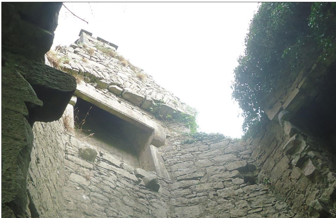
Plate 59: Ballintober Castle, northwest corner tower, view looking up to the third-floor fireplace in the north wall. The awkward alignment of the fireplace with the gable above indicates different building programmes. It is likely that the fireplace is the later addition
