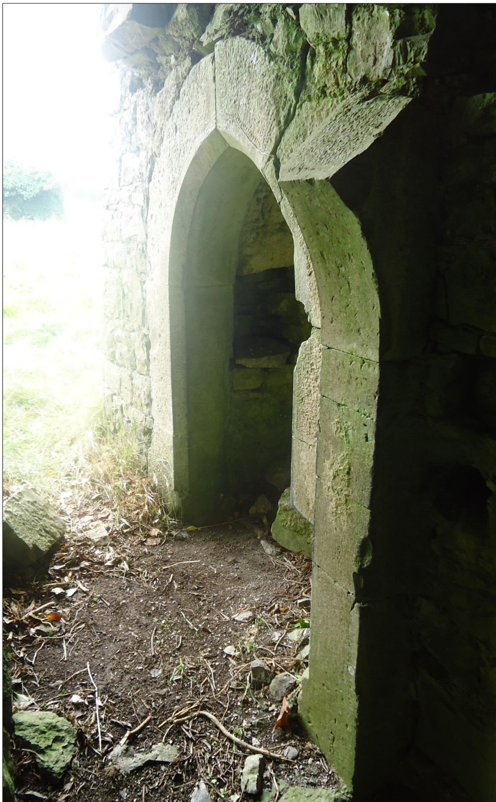
Plate 42: Ballintober Castle, northwest corner tower, view of doorway into stair passage, showing the nature of the doorway's construction, which is typical of the doors in this tower
