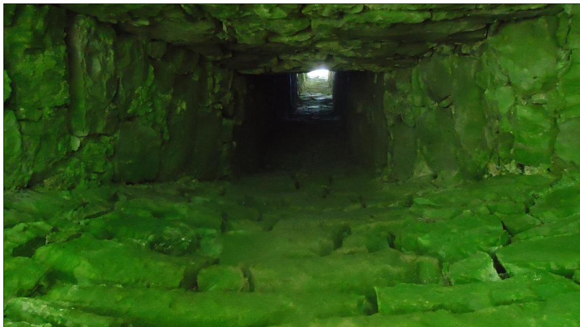
Plate 26: Ballintober Castle, southwest corner tower, view looking up the ground-floor chimney flue
