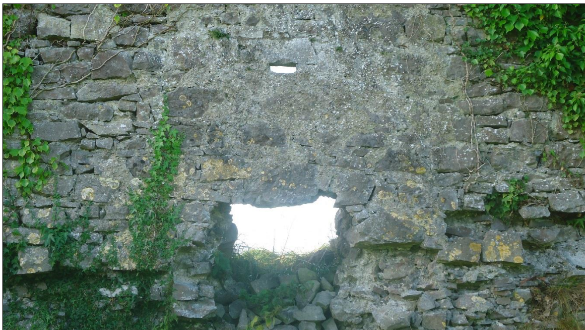
Plate 10: Ballintober Castle, view looking at the exterior of one of the gun loops on the north wall, showing render surviving around the opening in contrast to the wall fabric away from it, indicative of the inserted nature of this opening
