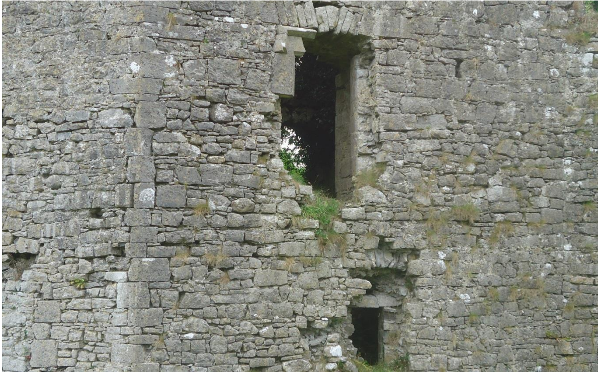
Plate 49: Ballintober Castle, northwest corner tower, external view showing the remains of the west-facing windows on the ground- and first-floor levels. Note too the quoin stones on the angle of the tower to the left (North) and the line of four quoin stones further left that mark the blocked-up ground-floor window in this angle
