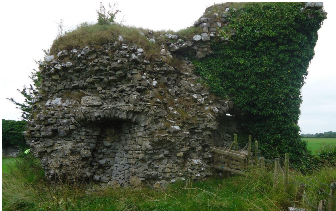
Plate 72: Ballintober Castle, eastern entrance, view of the north tower's interior, with the rear chamber to the left (West) and stone massing above indicative of vaulting, and front chamber to the right (East)
