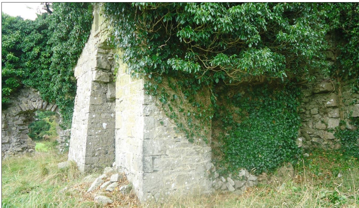
Plate 40: Ballintober Castle, northwest corner tower, view showing the buttressing added to the south wall to support the tower, presumably during the 19th century
