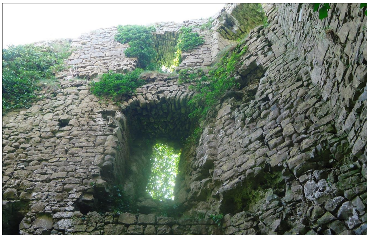
Plate 32: Ballintober Castle, southwest corner tower, view looking up at the first- and second-floor windows on the east wall
