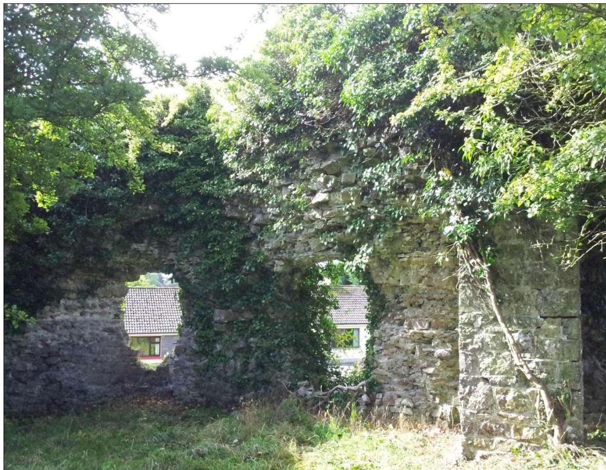
Plate 68: Ballintober Castle, southeast corner tower, view looking south, showing stone massing above the ground-floor openings, indicative of a vault structure. The vertical column on the right (West) side is a supporting buttress introduced presumably in the 19th century
