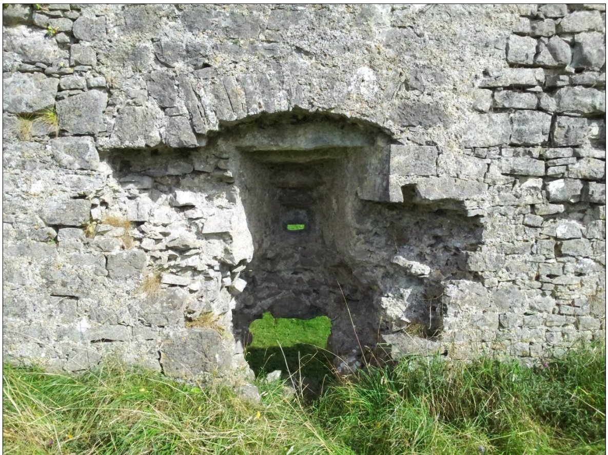
Plate 16: Ballintober Castle, view looking at interior of north wall showing gun loop with narrow rectangular hole, west of the mural stairs
