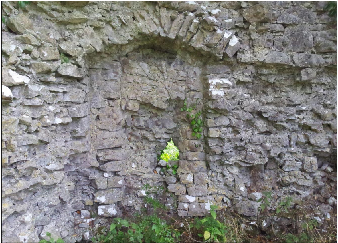
Plate 63: Ballintober Castle, northeast corner tower, view of reworked recessed opening in northeast angle of the ground floor
