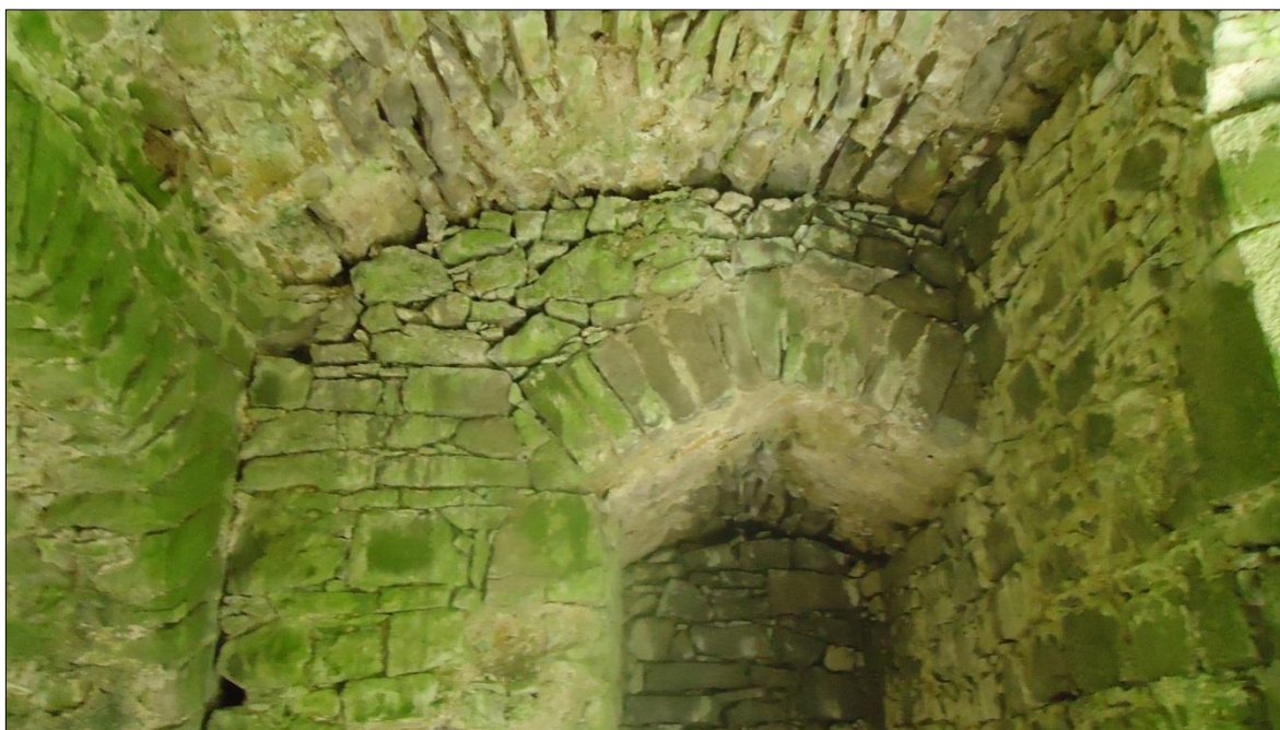
Plate 30: Ballintober Castle, north chamber in southwest corner tower, view looking north to the inserted garderobe wall on the left with its simple arch to form a recess to the right. The end/north wall of the recess is a blind for a second/primary garderobe chute behind it
