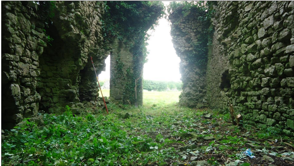
Plate 21: Ballintober Castle, view looking North from interior of the southwest corner tower, showing the ruined nature of the north wall and the presence of the buttress inserted to support the tower
