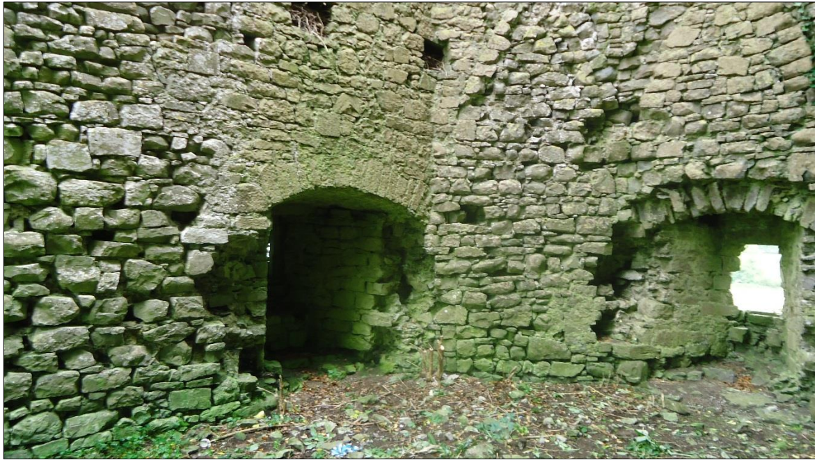
Plate 23: Ballintober Castle, southwest corner tower, view looking at ground floor window in east wall
