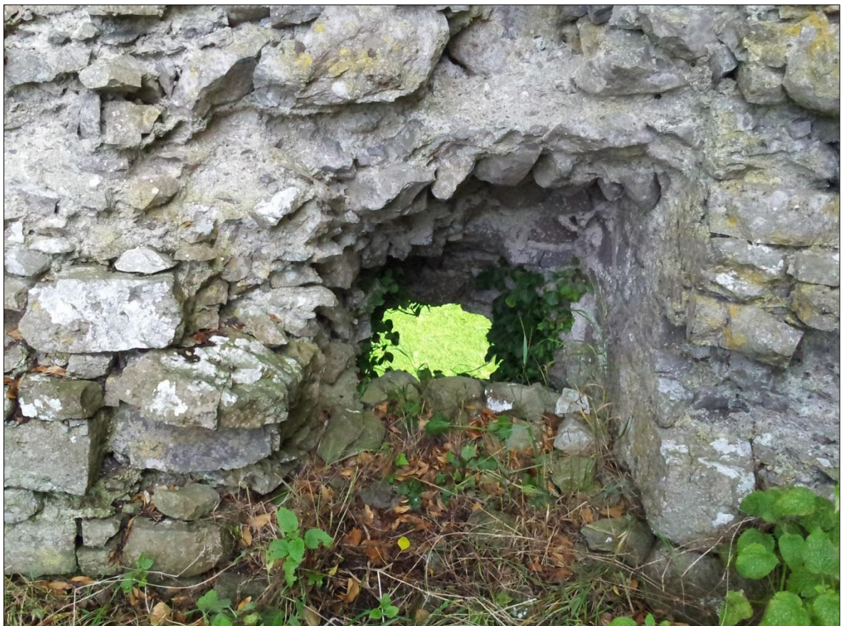
Plate 62: Ballintober Castle, northeast corner tower, view looking at the gun loop at ground level in the north wall
