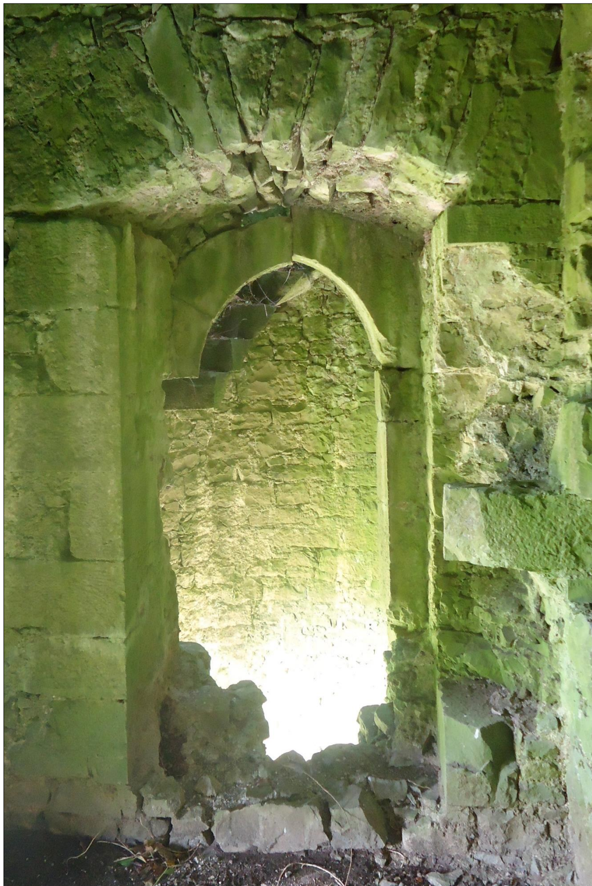
Plate 52: Ballintober Castle, northwest corner tower, view looking out (West) of the doorway into the mezzanine first-floor level
