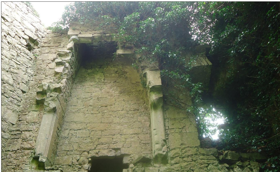
Plate 57: Ballintober Castle, northwest corner tower, view of the second floor showing the fireplace and window on the east wall
