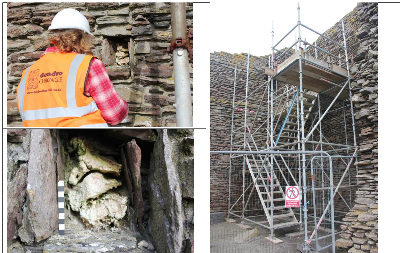
Figure 2 Clockwise from Top Left: Inspecting the timber, the scaffolding access, and the weathered outer face of the in situ timber before any intervention (Scale in 1cm intervals).
