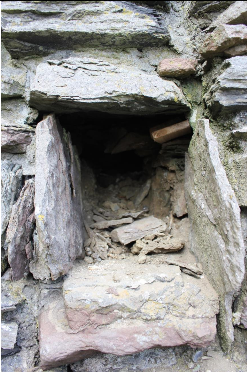
Figure 3 The socket after removal of the timber (note, the wooden wedge to top right is ours, and was placed in temporarily to lift stones off the top of the timber during extraction). It was removed prior to the socket being closed up by HES works team. Photo: C Mills 23.09.21.
