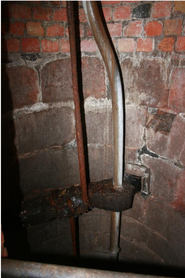
43 The shaft at inspection-chamber level showing the top brick courses and the pipe and unidentified iron rod retained by the uppermost wooden beam inserted into the stonework
