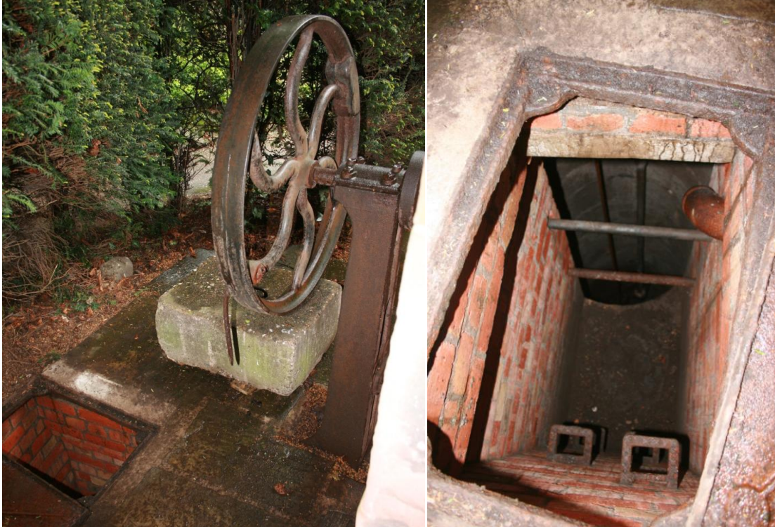
Left: 40 The pump in relation to the inspection chamber (the concrete block has just been moved off the inspection chamber cover); right: 41 The inspection chamber and well shaft
