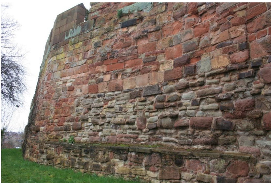
37. The north-west end of the north curtain wall, showing multiply rebuilt masonry above probable primary Green Coed-yr-Allt Beds sandstone slabby rubble
