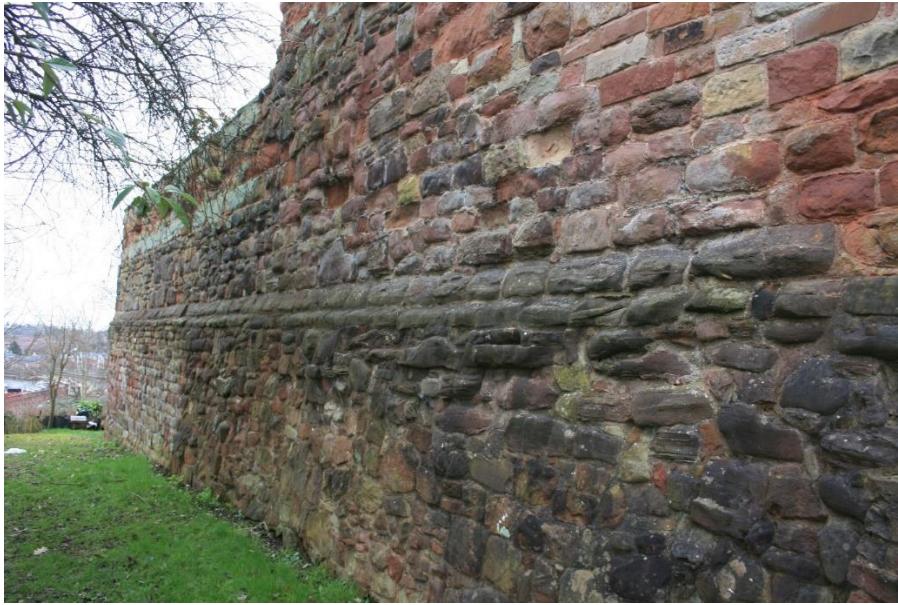
38. The central section of the north curtain wall. This marks the commencement of the sandstone rubble section with high plinth courses examined in Trench 4
