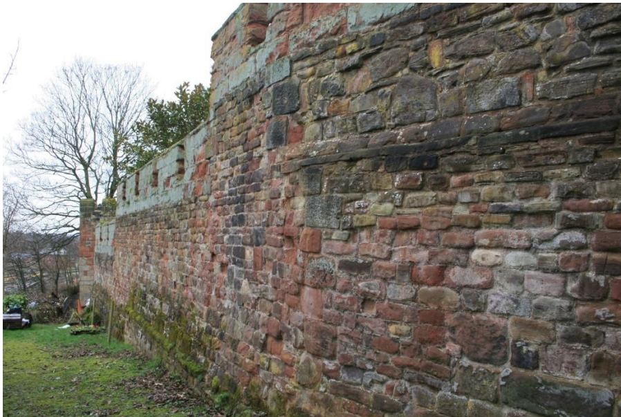
39. The east section of the north curtain running down-slope (the motte ditch profile) to the Postern Gate. Trench 4 examined this section
