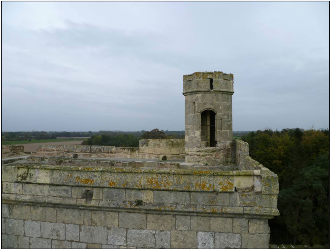
Plate 13: Stair turret opening onto roof leads of south-west tower, showing example of lower (rebuilt?) parapet walls, looking N.
