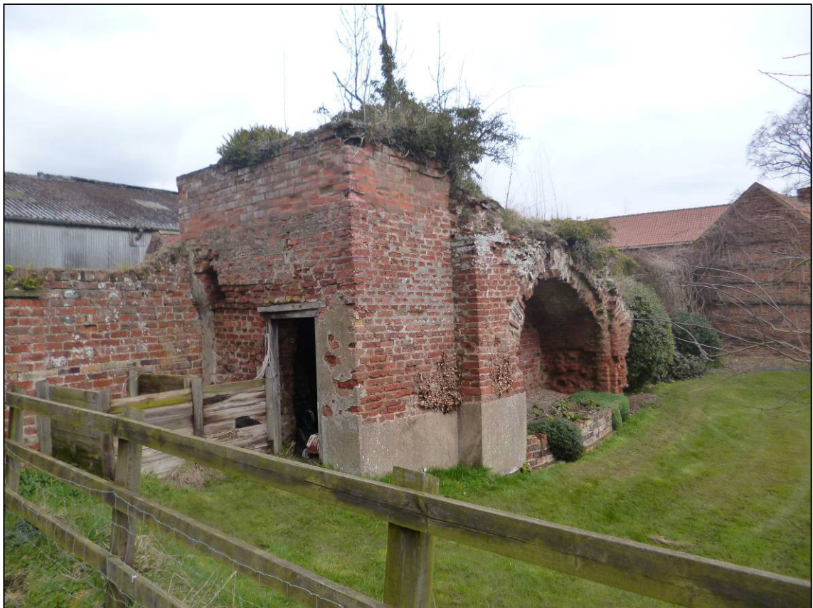
Plate 6: Brick structure (Site 2d) at north end of east moat (Site 2c), looking NE.
